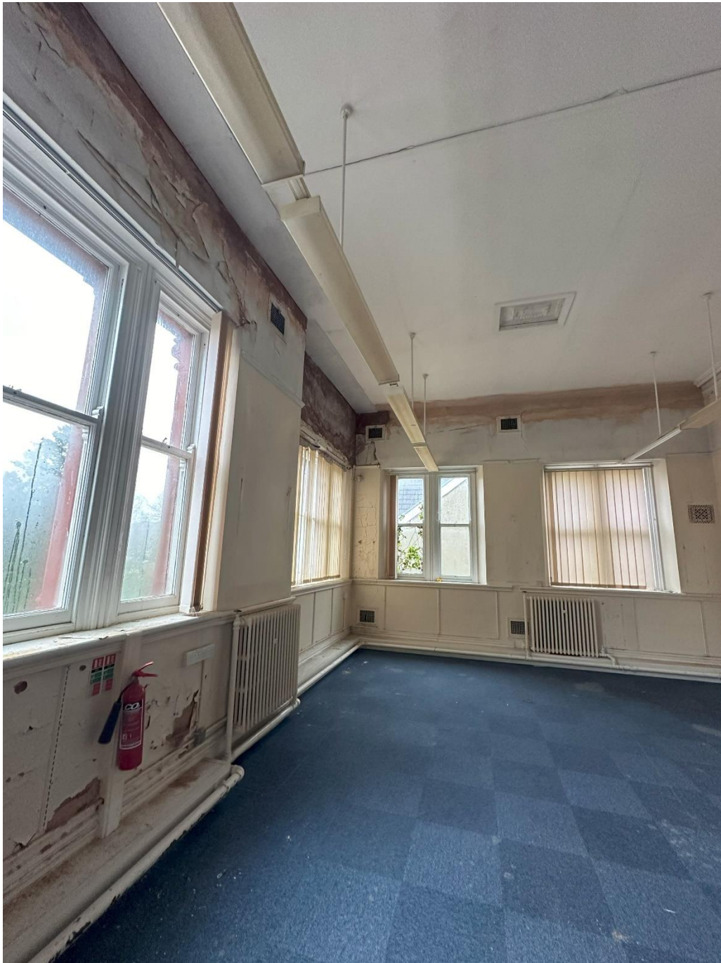
Figure 3: Photo showing areas of damp (left hand wall, particularly above the windows).
