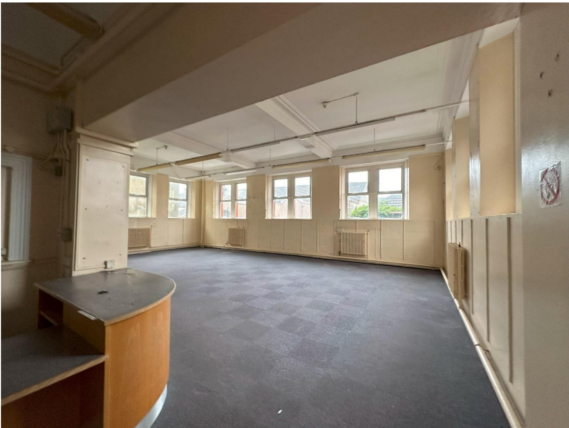
Figure 6: Ground floor main space, showing the light, airy floorplates and need for general refurbishment.
