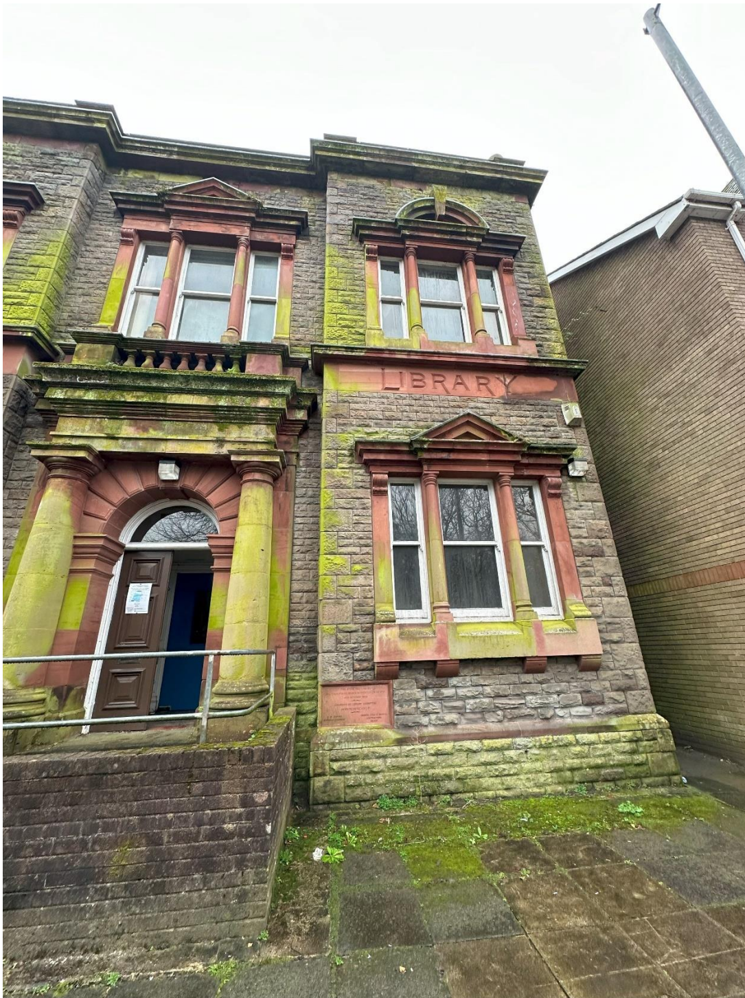
Figure 4: Main facade, showing need for external cleaning.
